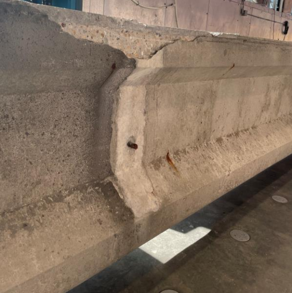
Rear end diaphragm sawcut damage (left side)
