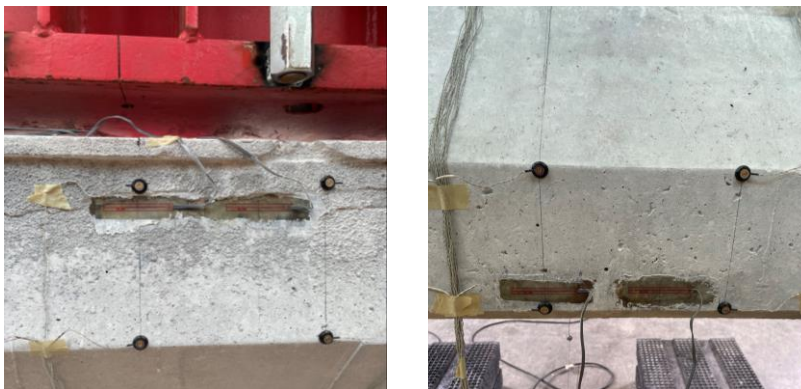
Figure B.23: Strain gauges at the top (left) and bottom (right) of a girder.
