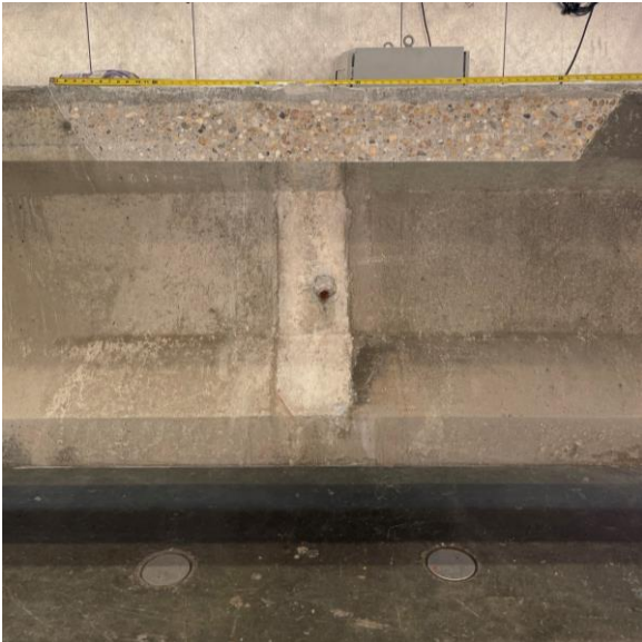
Front end diaphragm sawcut damage (left side)
