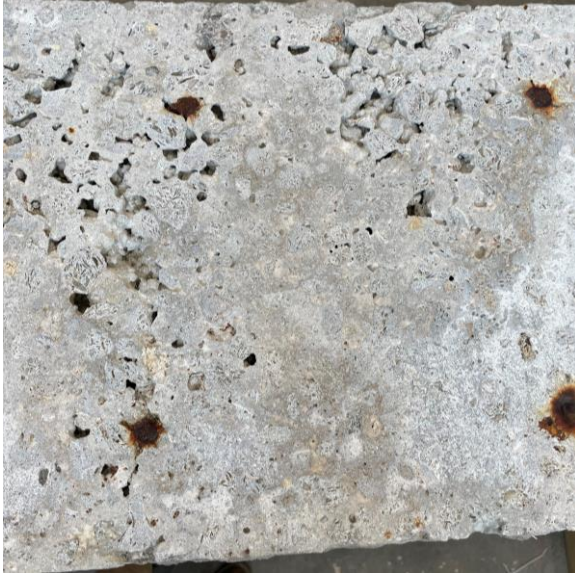
Rear deck honeycombing (top)
