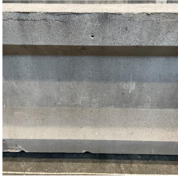
Spalled concrete (right side)
