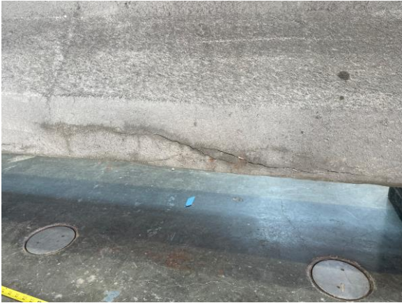
Front end bottom crack (left side)
