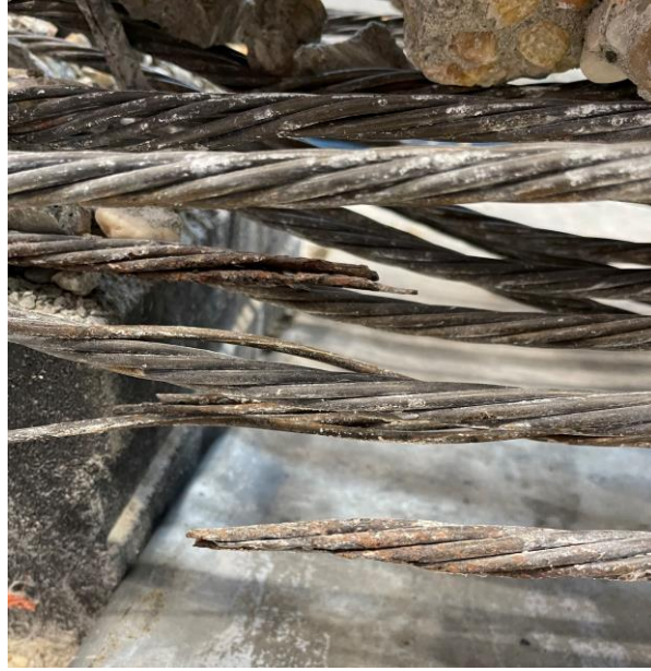
Figure 3.5: BTE1 corroded strands (visible only after testing).
