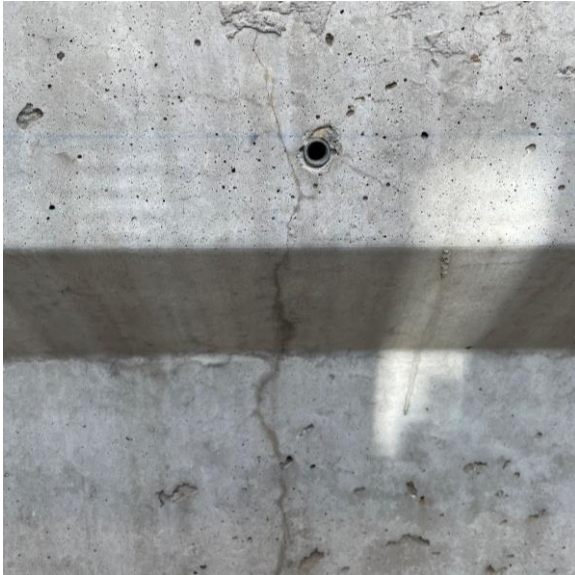
Midspan top cracking (right side)
